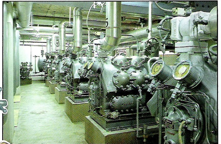
HC-800 compressors in a Danish slaughterhouse.
