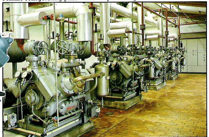
Fish freezing plant with HCT-125.
